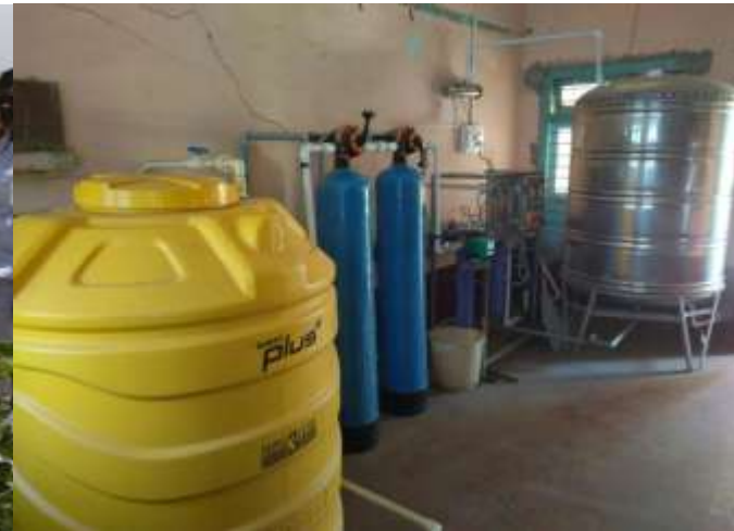
Over Head Tank and RO Water Purifier Durgamba High School, Davanagere
