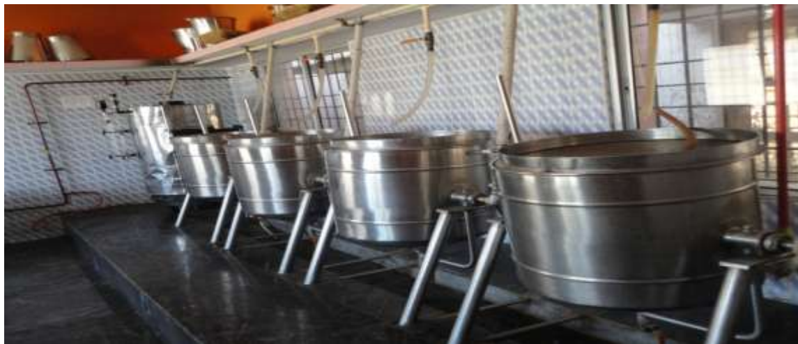
Steam Boilers are being used for Cooking MDM at Govt HS Basavanhalli, chikkamgalur Taluk & District
